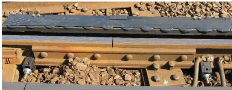
Figure 6. An example of the wayside lubrication system for restraining rail[10]
