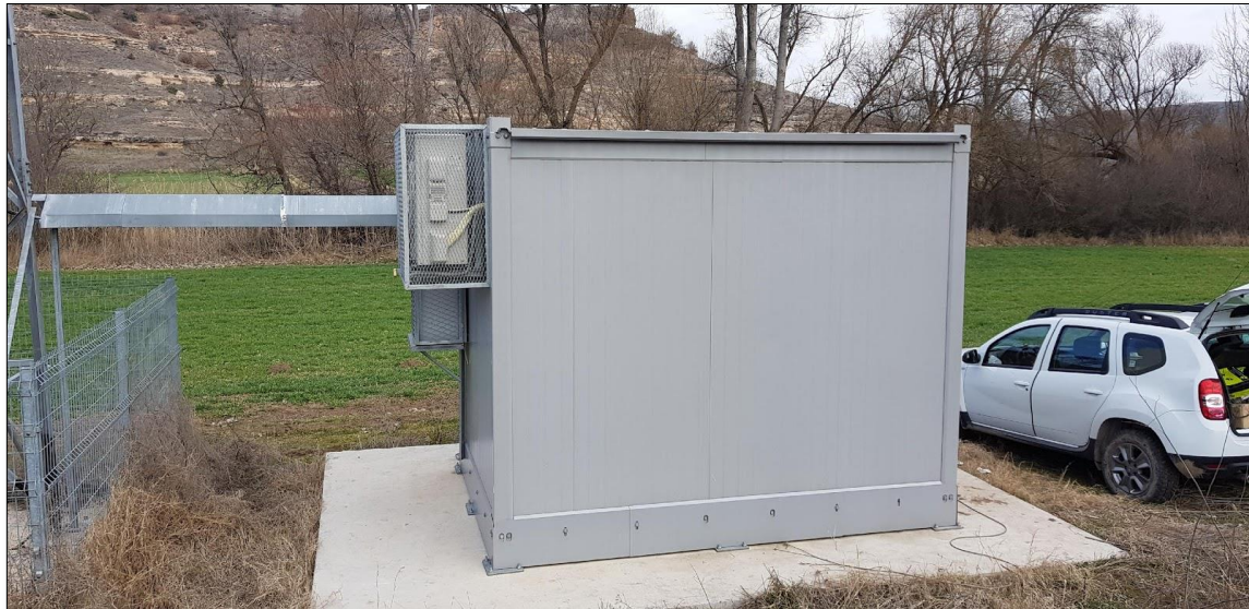
Figure 3.1.4 The signalization cabinet used for supplying electricity (220 V) to the test equipment
