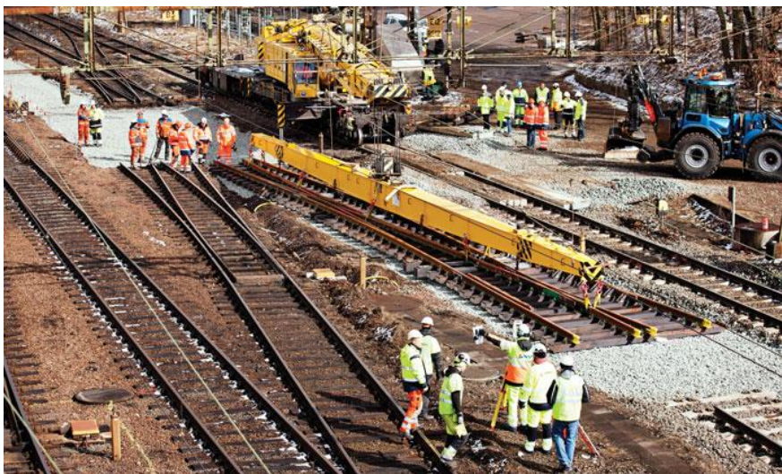
Figure 2.5 - Example of crane able to lift S&C sections whilst under overhead lines. 2
