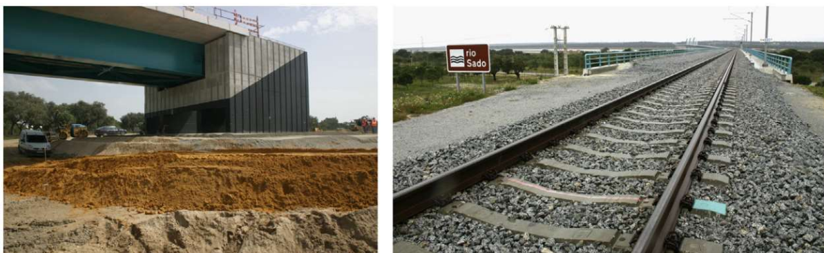
Figure 14: Side view of the transition zone before construction and general view of the track [4]
