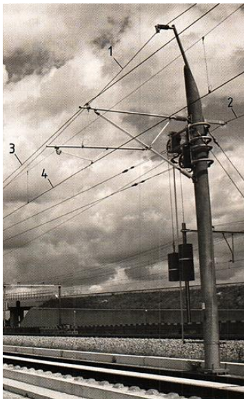
Figure 4.24 - Contact Line arrangement on an interstation section of the HSL Zuid line; 1 - negative feeder; 2 - return conductor; 3 - catenary wire; 4 - contact wire.
