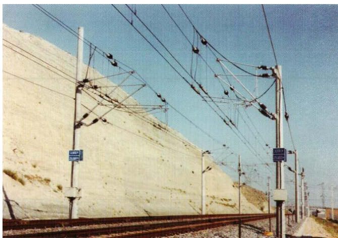
Figure 4.15 - Madrid-Seville high-speed line, neutral section between DC and AC power supply, Spain
