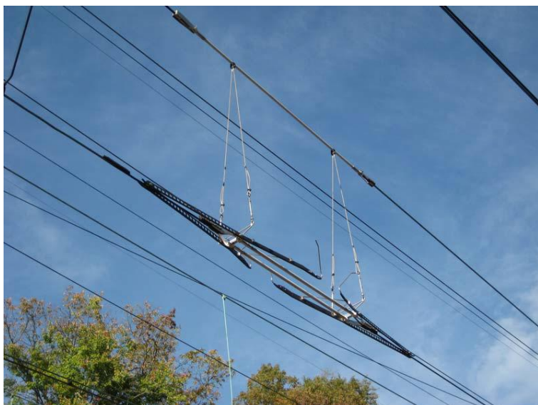
Figure 3.15 – Neutral section insulator
