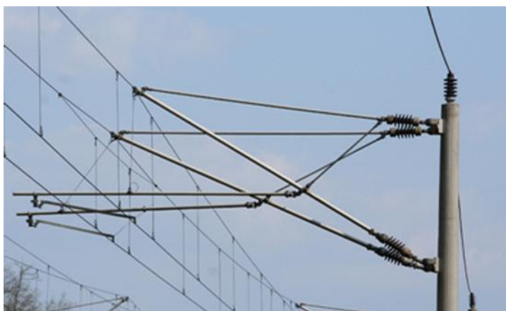
Figure 4.33 – Compound overhead line 13
