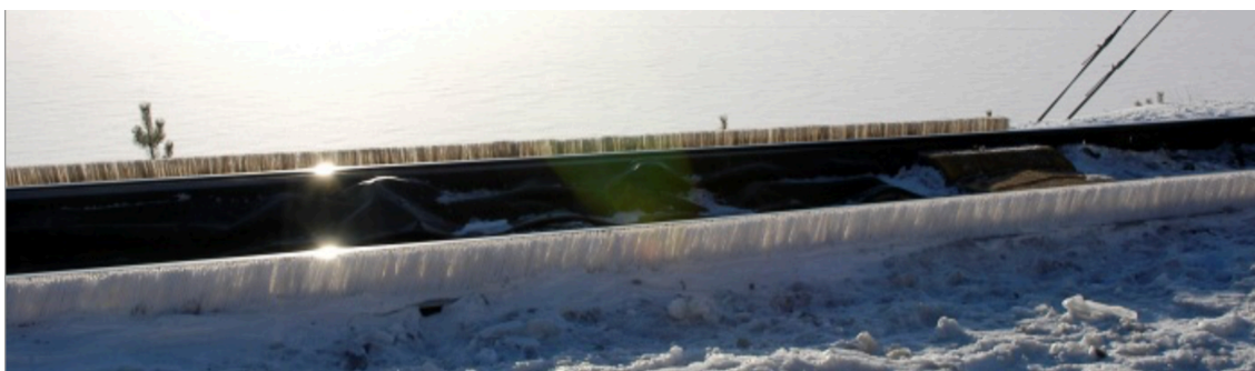
Figure 3.6 - A track equipped with SnowProtec (Vossloh, 2014)
