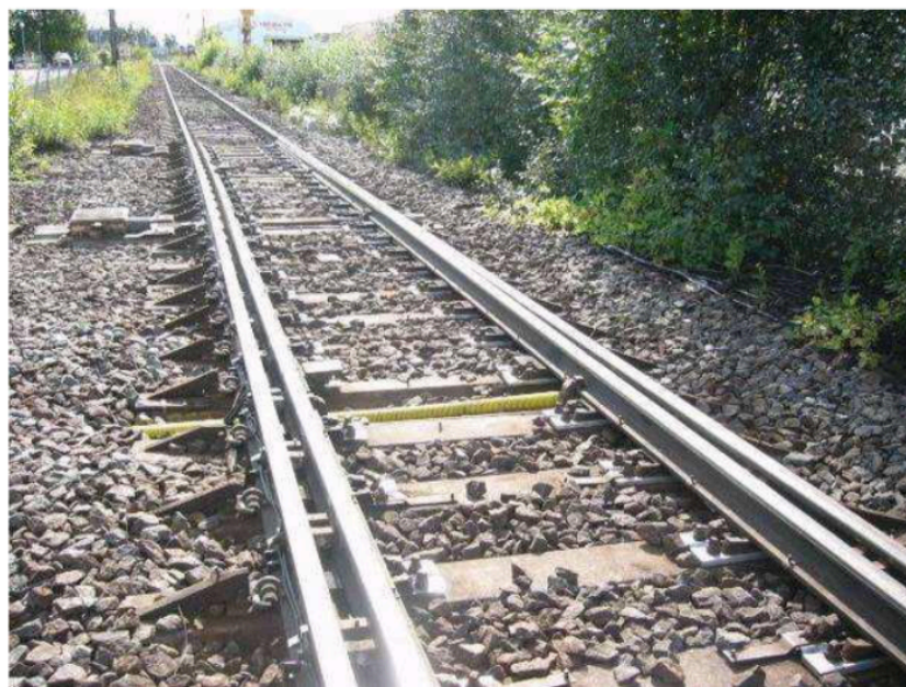
Figure 3.3 - SwedeSafe on a railway (Enno Wiebe, 2010)
