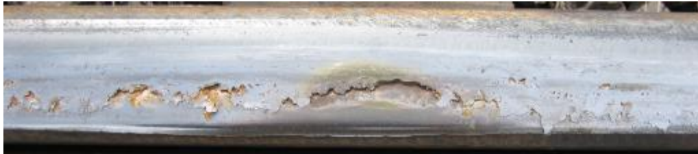
Figure 1.14 - Burning of Rail 10
