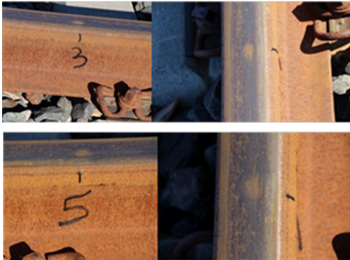
Examples of some of the defects detected.
